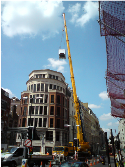
The installation in Central London
