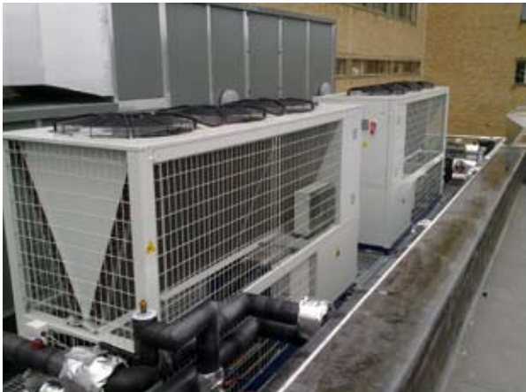
2 Taurus Tech 055/SSN chillers
