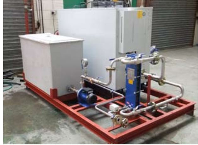
The completed cooling package on-site
