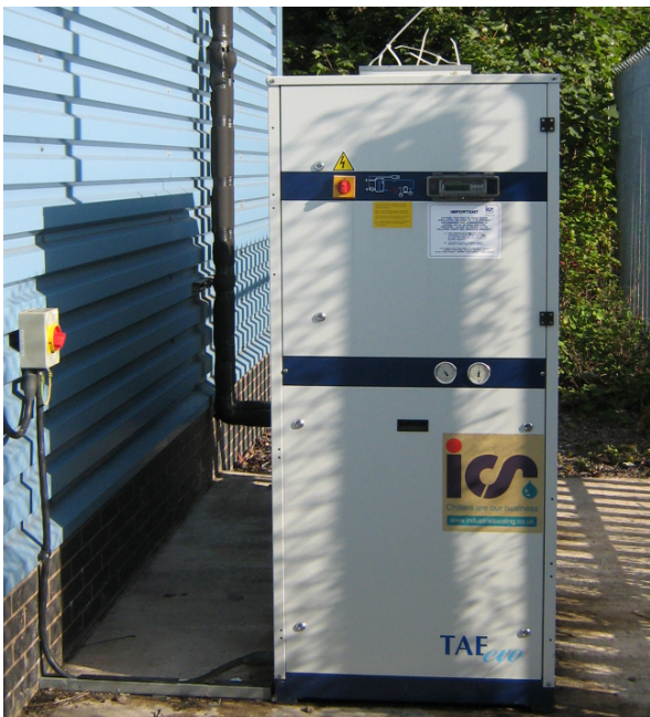
TAEevo 121 supplied to fit into existing footprint
