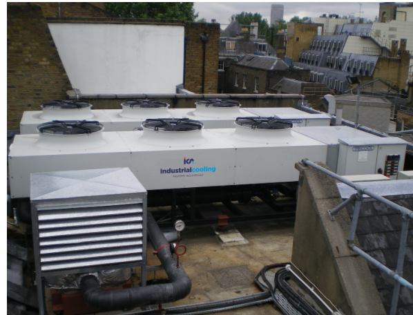
ICS custom built low profile chiller
