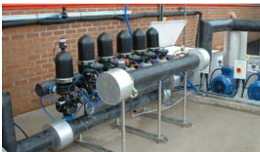
The Filtration System
