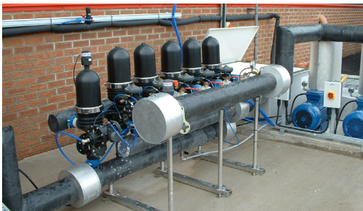
The Filtration System
