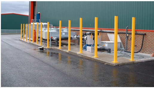
The Free Cooling System on site
