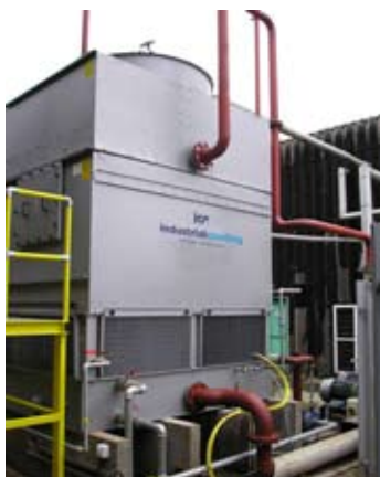
The Cooling Tower on Site
