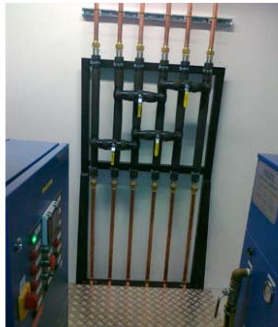
Typical arrangement of an open framed manual changeover panel shown above
