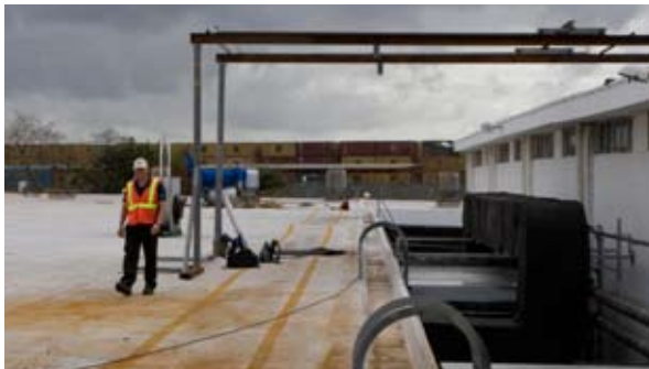
The new Air Handlers on the roof
