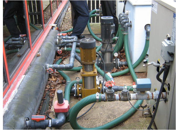
The non-ferrous pipework avoids contamination in the system
