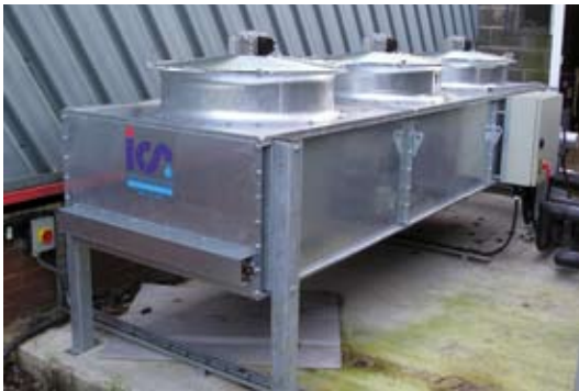
The Energy Saving Chiller On Site
