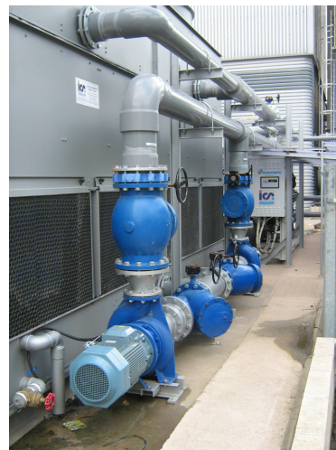
The Cooling System on site
