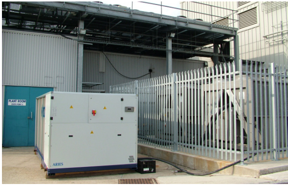
Cool Energy 250kW rental chiller supplied during the retrofitting of an R22 Chiller.
